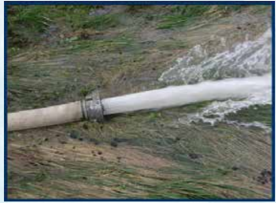
After 26 hours the rinsing was stopped. The water was clear and the pipes were clean!
